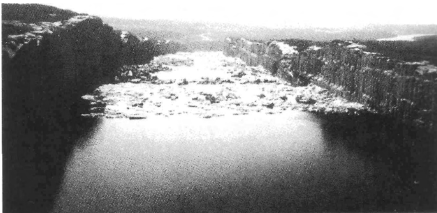
The view from the top of the huge spillway. The outlets of the generators from La Grande 2 and 2a are where the river is visible in the upper right. The height of the stone face sidewalls is about 60 feet.
