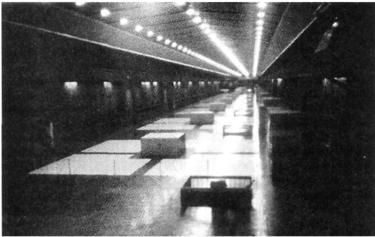
The LG2 generator hall. The tops of 16 generators are visible.
