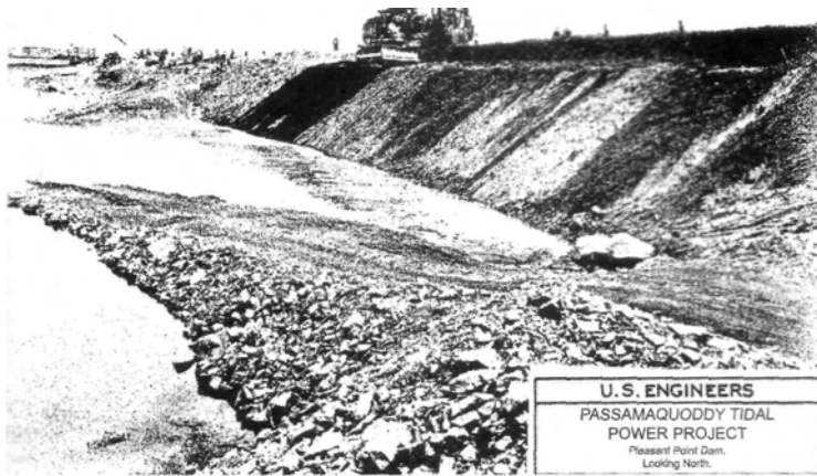
Pleasant Point Dam, part of the plan for the Passamaquoddy Tidal Power Project, under construction in 1936. Courtesy Eastport 200 Committee
