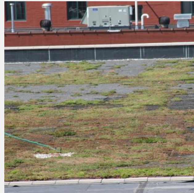
Bare Spots – Green Roof Technology, 2017
