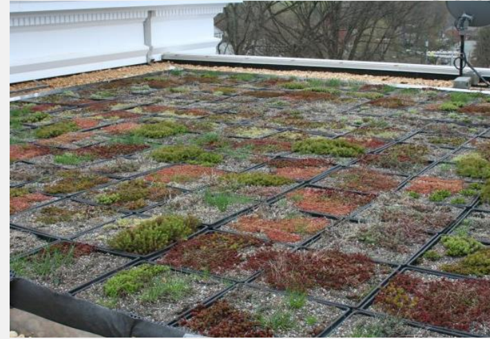
Bare Spots – Green Roof Technology, 2017
