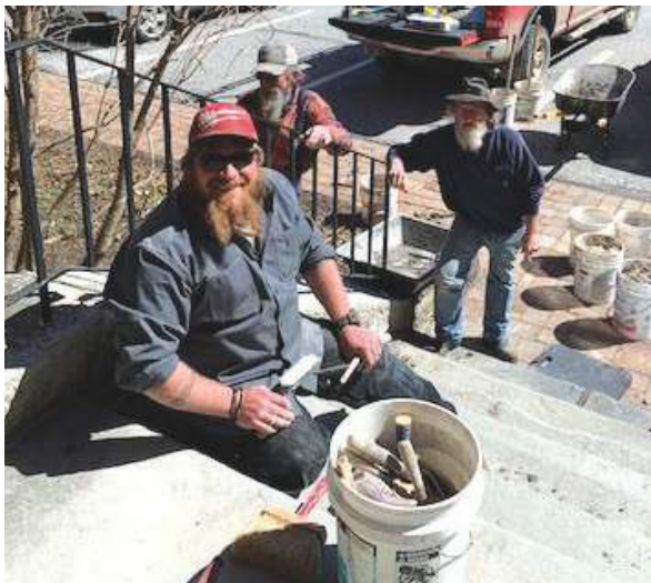
Cody Surething, Randy Parry, and Fred Decelle complete masonry on the front stairs of the Black River Academy Museum.
