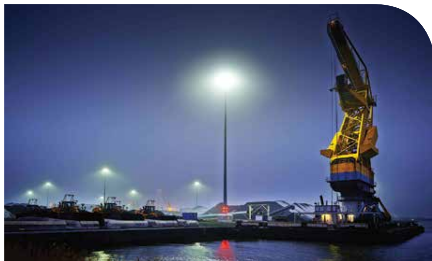
PORT AMSTERDAM RIETLANDEN: AAA-LUX is the first manufacturer that manages producing sufficient light with LED's from 45 metre height.
