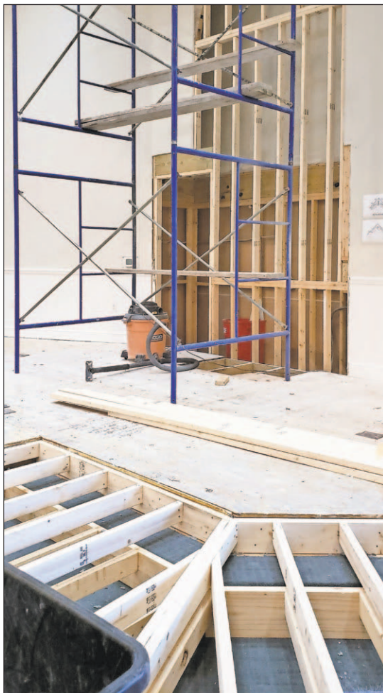
The former altar/stage has been extended from the dais that Town Council and the town clerk will sit at during meetings at the new Town Hall.
