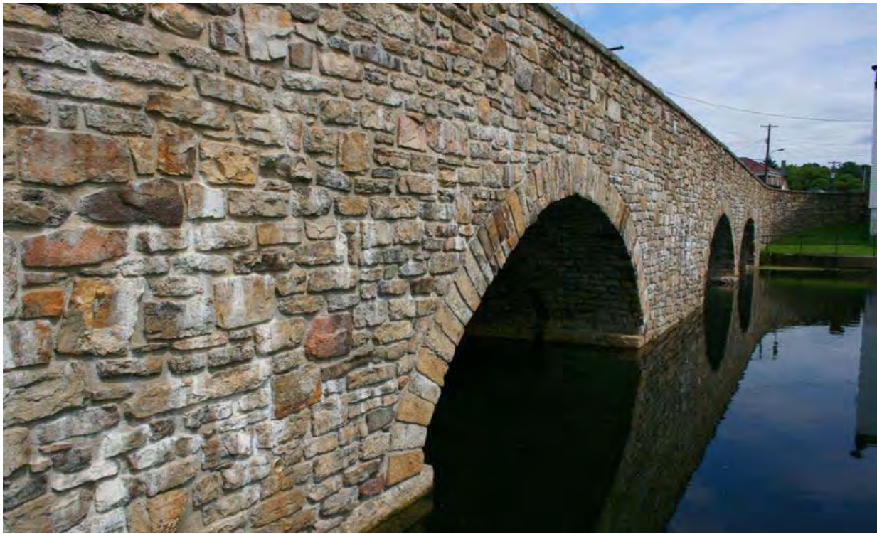
Fig. 6 Lyndhurst Bridge, built in 1856-57. The stone is mainly Potsdam sandstone, but some fieldstone boulders and cobbles of granite, gneiss and gabbro have been incorporated.
