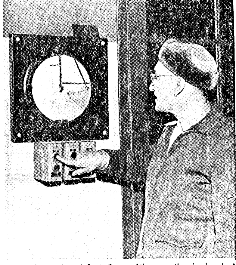
Well controls and Supt. George Allen . . . the circular chart at left charts the reservoir water level throughout a 24 hour period. The controls are located in light plant. Workmen can cut in one of both wells.
