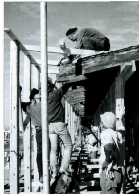
Work crews repair the façade of Kit and Maria Josefa Jaramillo Carson's home. The project, completed in November 2001, was partially funded by a federal grant. Photograph by Victoria Jacobson.
