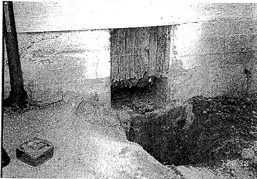
Photo No. 14 Decayed Bottom of Column
