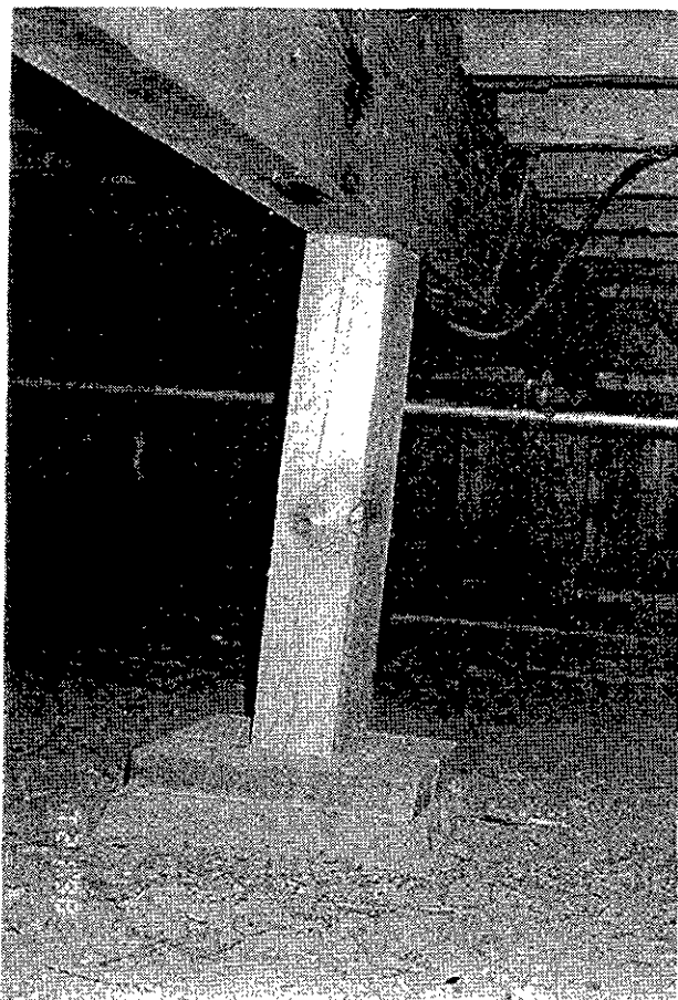
Photo No. 15 Floor Beam, Post and Footing in Crawl Space of North Wing
