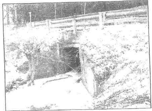
Figure 3: Poor condition box culvert
