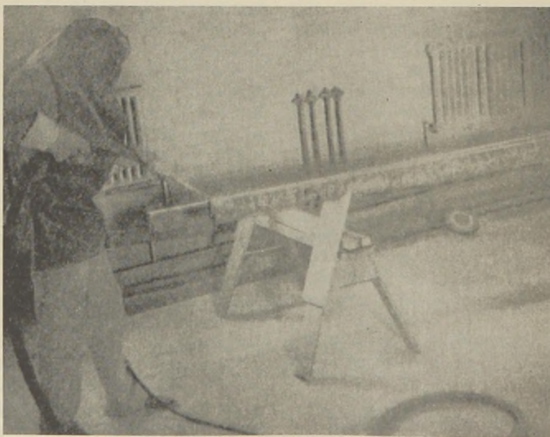
FIGURE 1.—Sandblasting metal equipment parts prior to zinc metallizing at the Fort Dodge, Ia., sewage treatment plant.
