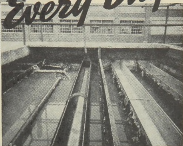
Settling Tank for the settling of coagulated wastes; showing one flight, chain, sprocket and shaft of L-B Sludge Collector; Roto-line scum skimmer; baffle board and troughs for run-off of treated waste water. Water level lowered to show equipment.
