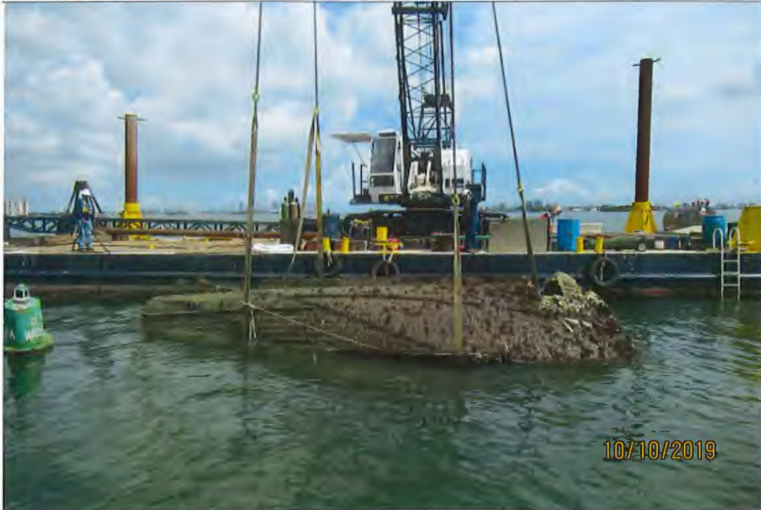
Sunken vessel hull being removed from edge of ICW. Note damage (at right) from recent vessel strike.
