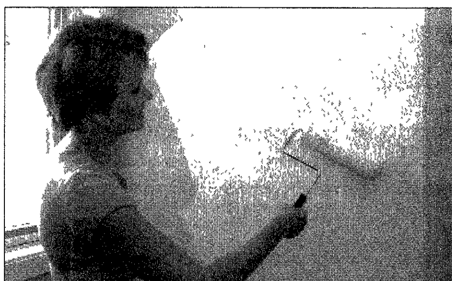
Many apartment communities allow residents to paint their apartments in neutral tones.
